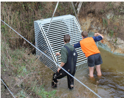
Adam and Daniel Hall installing the one-way pest fish barrier over the culvert at the outlet to Lake Ohinewai. The purpose is to let fish out but not allow them to return. The trap can be cleared of debris by lifting the gate. Photo: A. Gray
